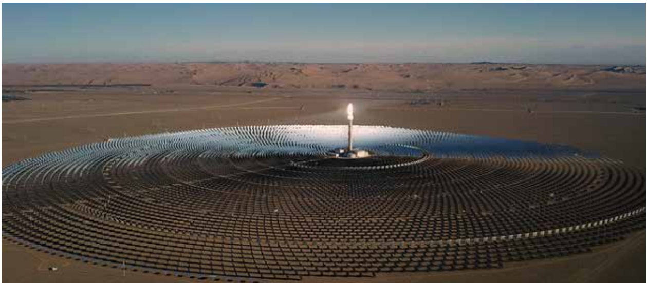
The heliostats of a molten-salt solar thermal power plant in Dunhuang, in northwest China's Gansu Province, on Oct. 23, 2019.
