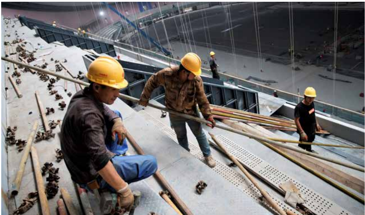
Construction workers built Beijing’s new National Speed Skating Oval on September 23 – one of many infrastructure projects being built in China.
